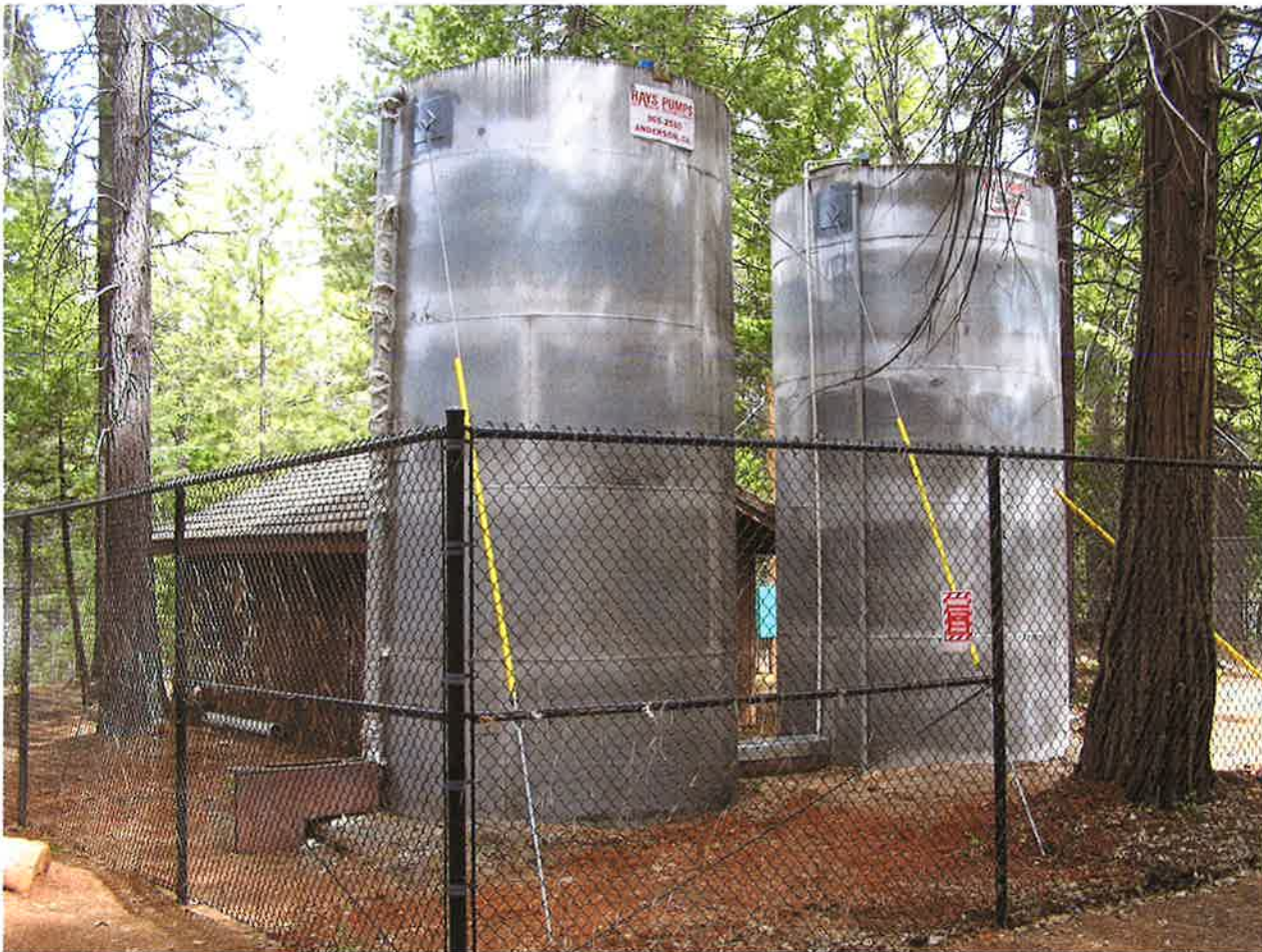
Two Existing 9,000 Gallon Tanks
