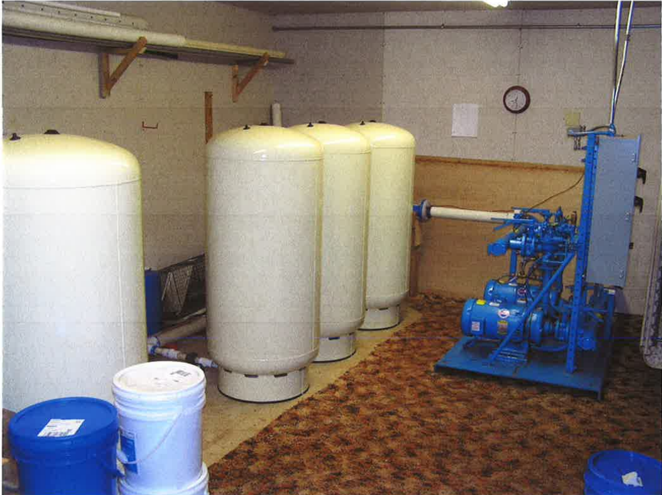
Existing Booster Pumps and 4 of 6 Hydro Pneumatic Tanks
