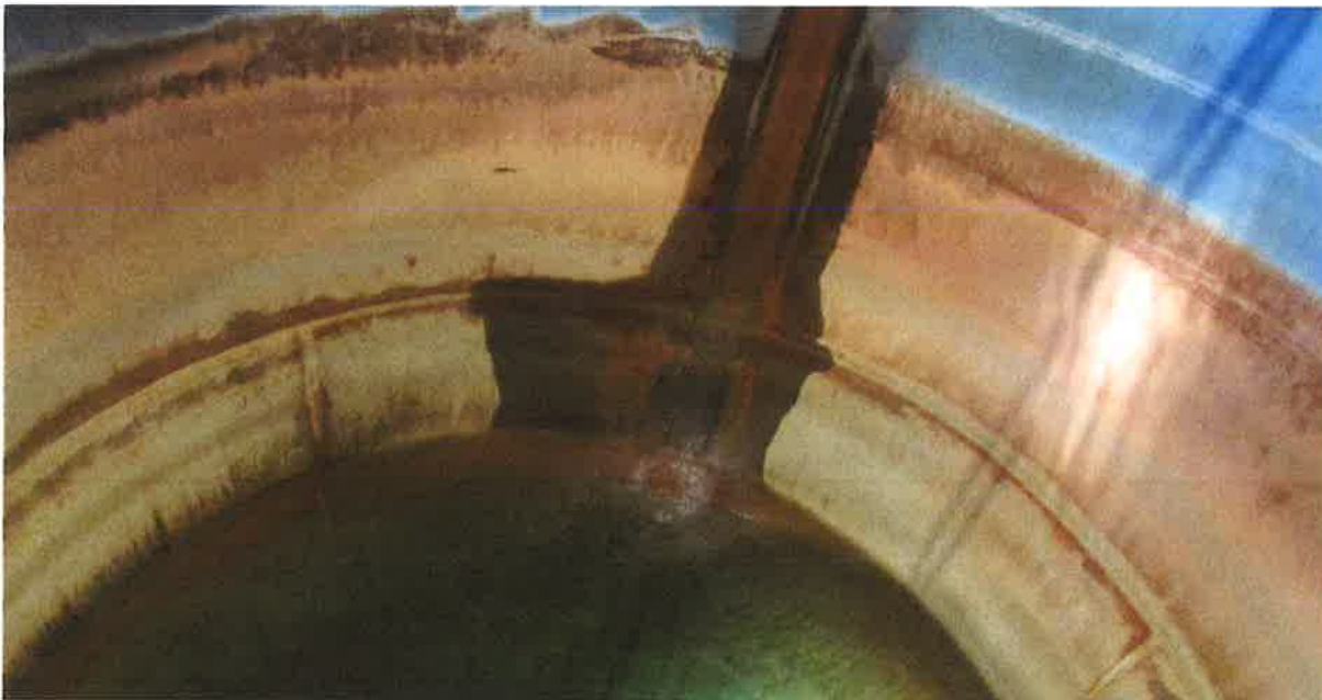
Rusted Interior of Storage Tank
