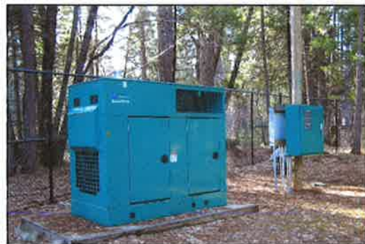
60KW Standby Generator
